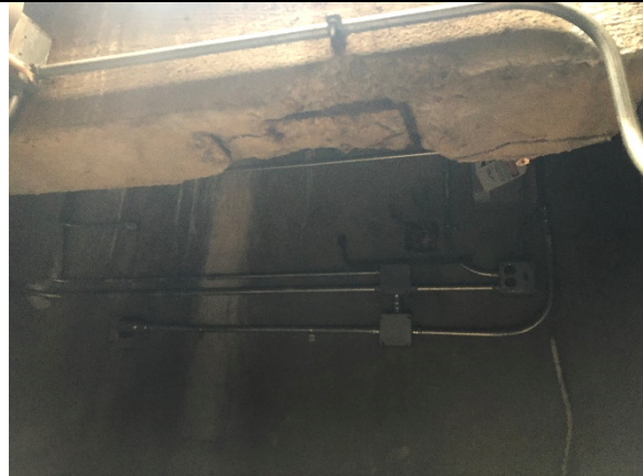
Figure S-16 Exposed Rebar in Beam at Loading Dock
