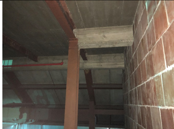
Figure S-7 Steel Framing in Attic with Minor Corrosion
