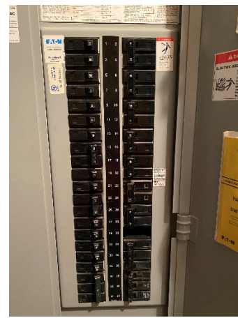
Missing blank covers over spares
