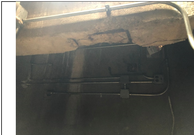
Figure S-16 Exposed Rebar in Beam at Loading Dock (BSWL-B00BSE-001)
