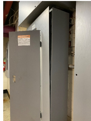
Panelboard with damaged door
