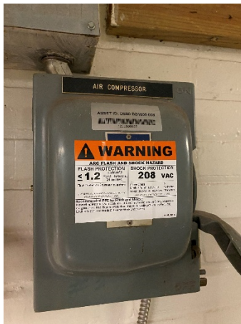
Disconnect Switch with nameplate data covered
