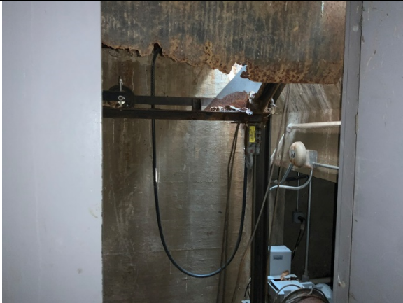
Figure S-15 Loading Dock Lift Equipment
