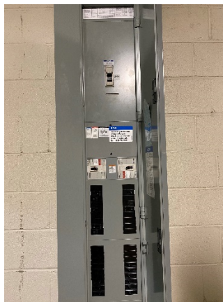
Missing number identifiers
