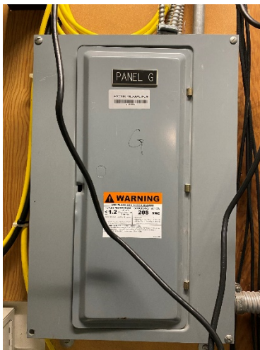
Panelboard with missing latch/lock
