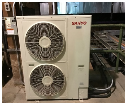
Outdoor Condensing Unit
