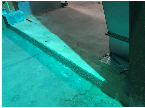
Figure S- 9 Crack in Topping Slab Curb (FDSL-B04000-001)
