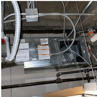
FPB missing filter
