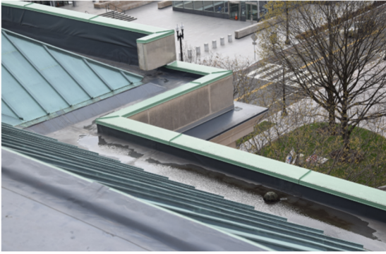
Standing Water by drain location
