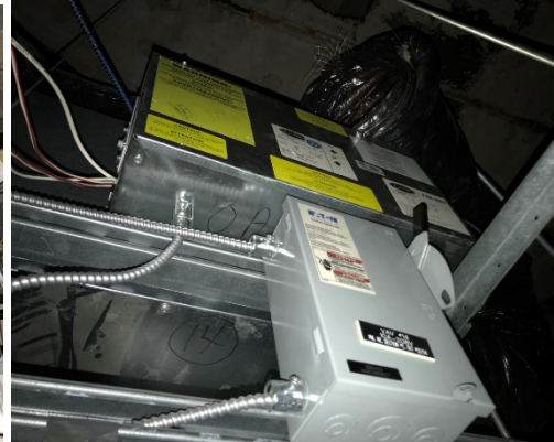
FPB primary air duct disconnected
