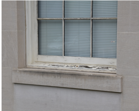
Wood Trim and Sill Condition at South Elevation
