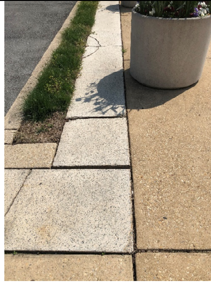
Figure S-19 Typical Settlement Cracking
