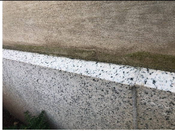
Figure S-12 Small Spall in Limestone at Base of Wall
