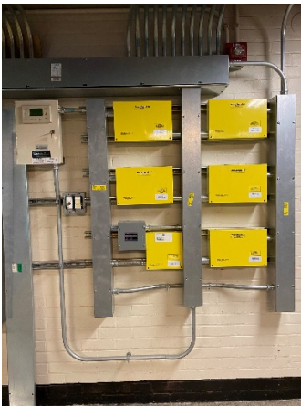
Lighting Control Panel
