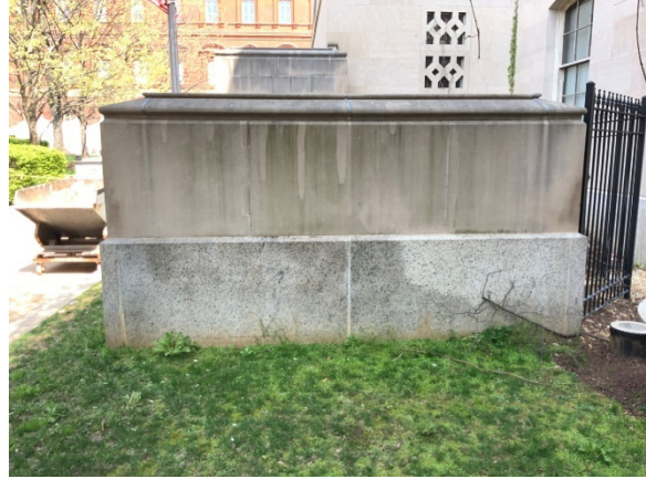
Figure S-14 Staining of Exterior Site Walls
