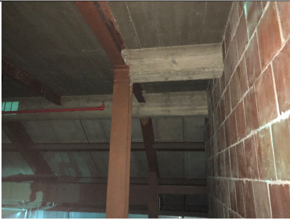
Figure S-7 Steel Framing in Attic with Minor Corrosion (RFR0- BR1000-001)
