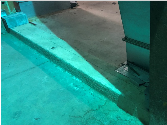
Figure S-9 Crack in Topping Slab Curb
