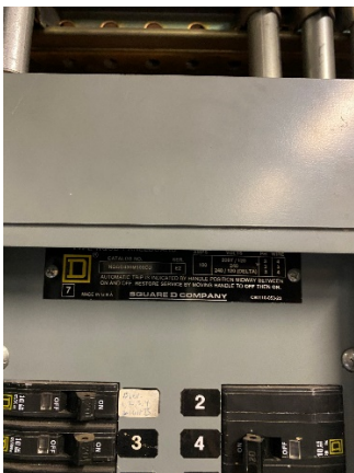
Missing front cover id label
