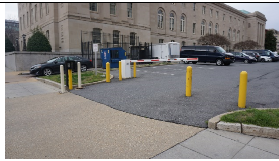
Vehicle Entry Control System, South
