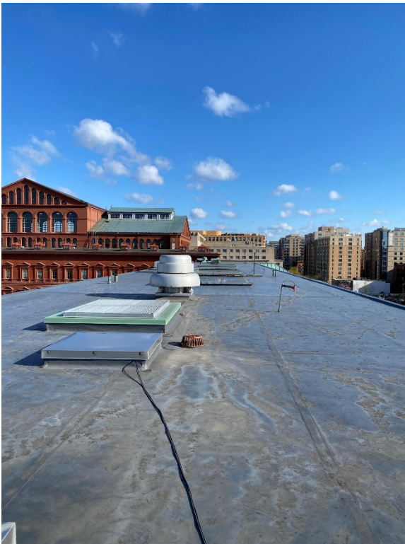
No lightning protection system
