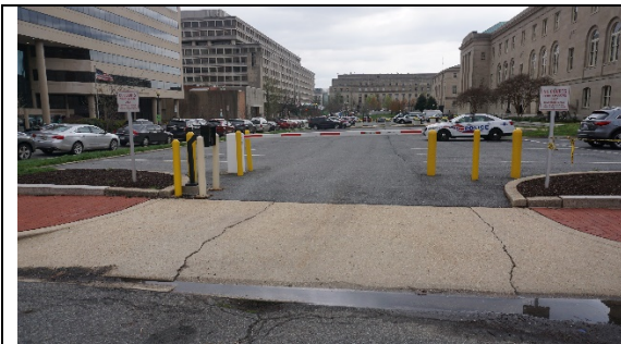
Vehicle Entry Control System, North
