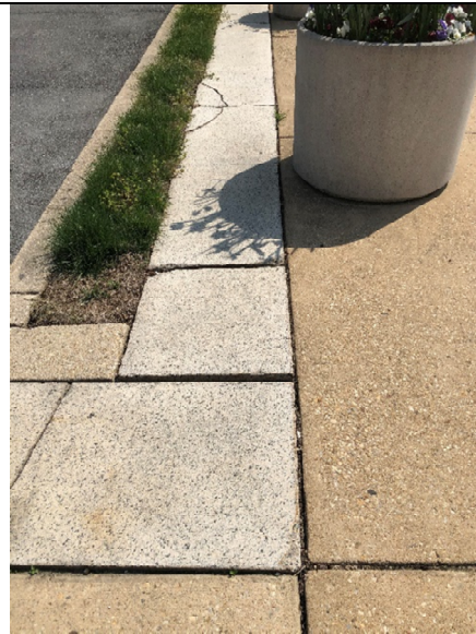
Figure S-19 Typical Settlement Cracking (PASU-B01000-001, PASU-B01SNE-001, PASU-B01SSE-001) (CGCG-B01SNE-001, CGCG-B01SSE-001, CUGU-B01000-001)
