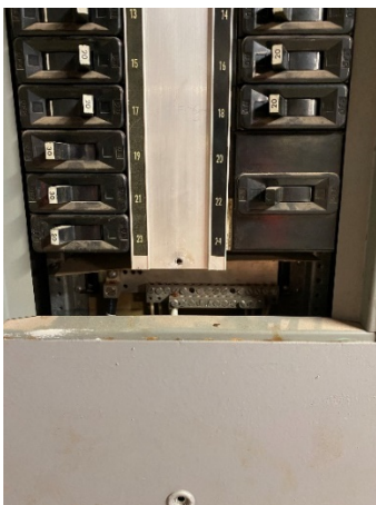
Missing interior face
