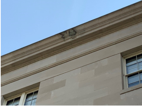
Figure S-13 Staining of Cornice Stone
