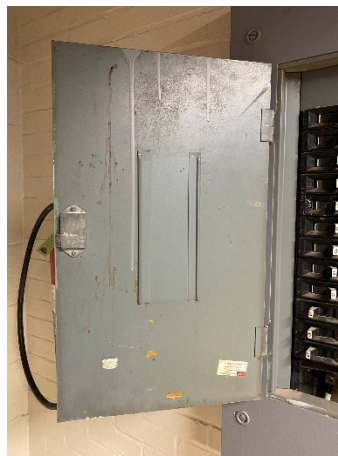
Missing circuit index card
