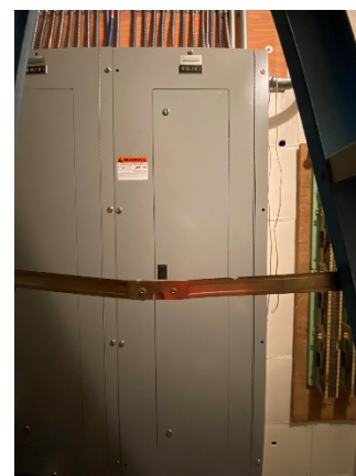
Obstructed working space
