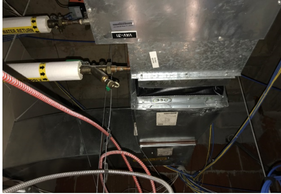
Typical Fan Power Box
