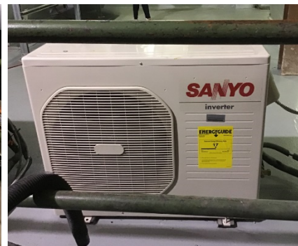
Outdoor Condensing Unit
