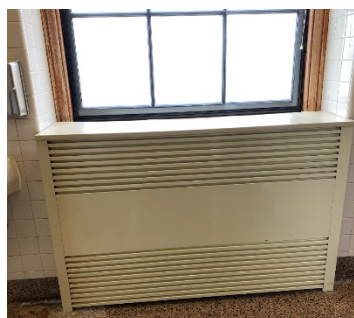
Restroom Steam FTR
