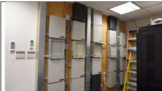
Card Reader Control Panel Assemblies
