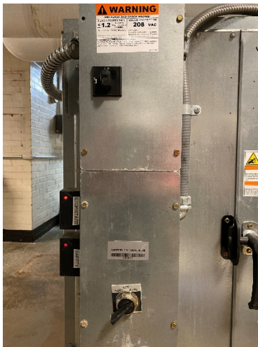
Rust & water damage
