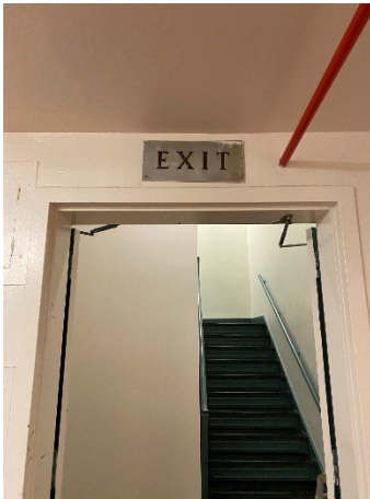
Unlit Exit Sign
